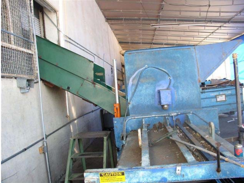
Exhibit 5. The feed chute with side panels missing and the three-foot step ladder used by the victim.
