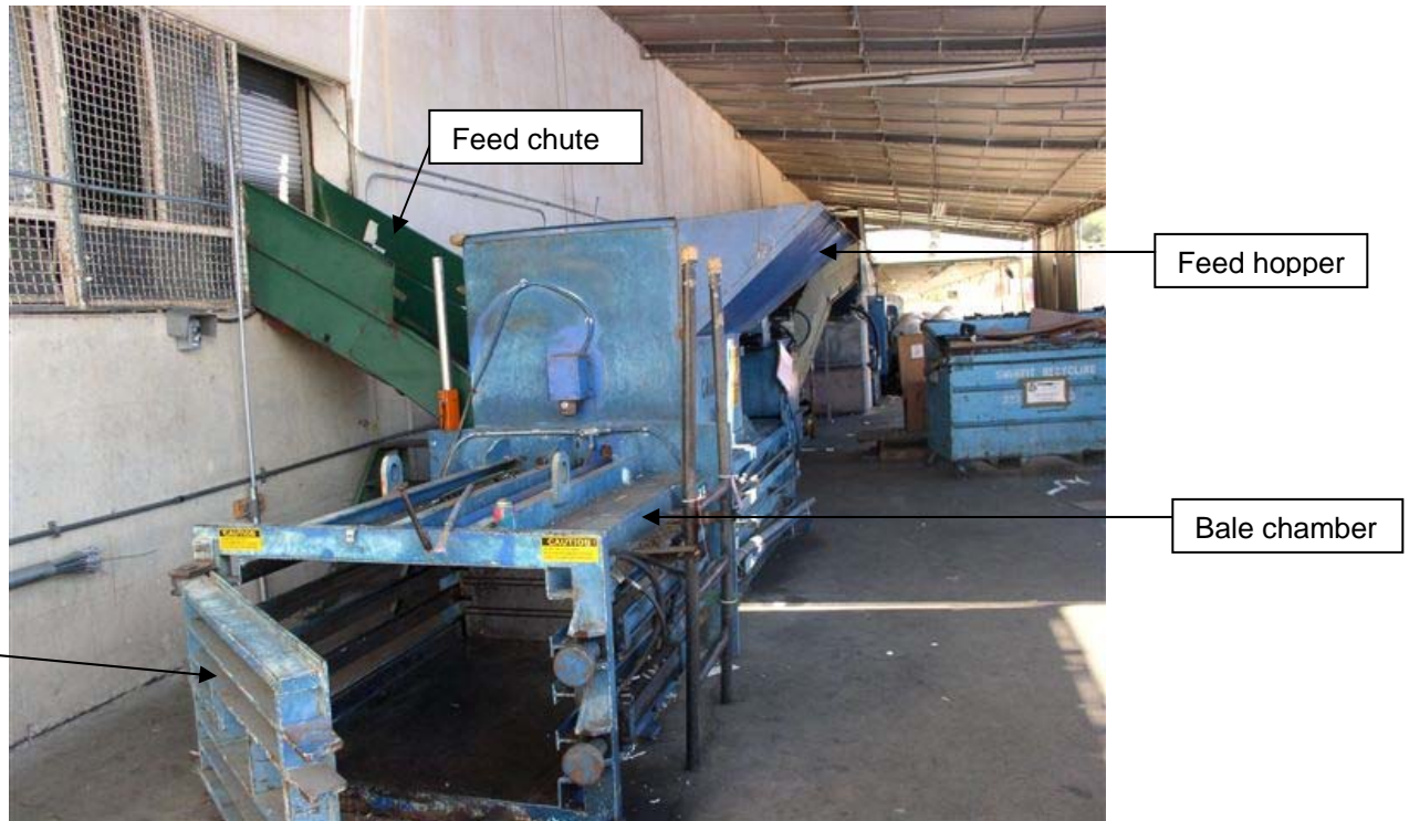
Exhibit 3. The cardboard baler showing the feed chute and chamber where the recycled bales of cardboard were formed.
