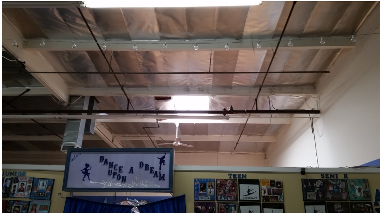
Exhibit 3. The dance studio theme room skylight opening involved in this incident.
