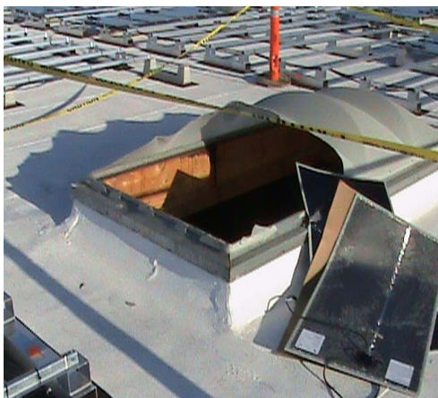
The skylight that the worker fell through
