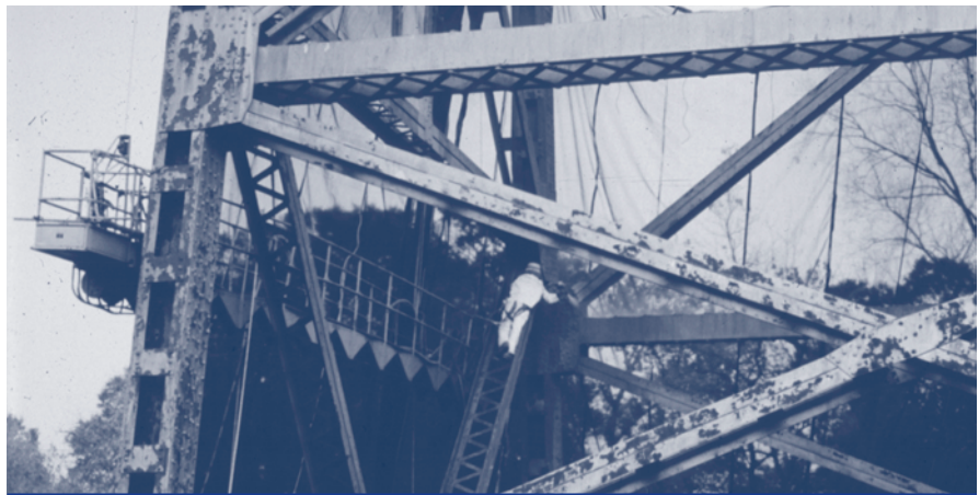
Industrial painters remove coatings with high levels of lead and chromium
